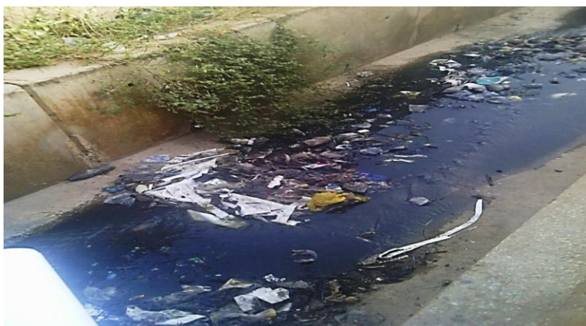
Fig. 2. Indiscriminate disposal of waste in Tunga Area of Minna Metropolis.
